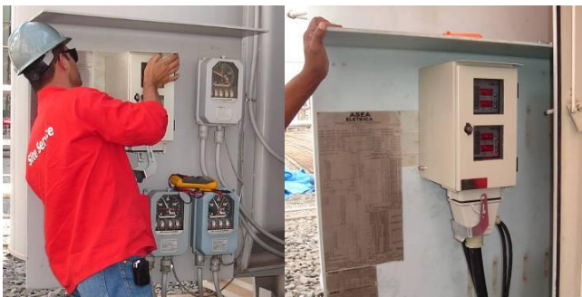
Figure 7 - Replacement of mechanical thermometers of the converter transformers for digital temperature monitors for the online monitoring system.
