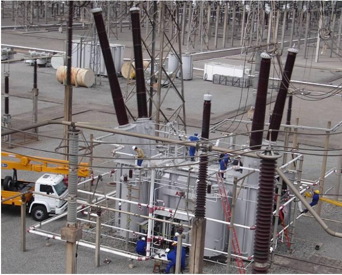
Figure 6 – View of a single-phase converter transformer
