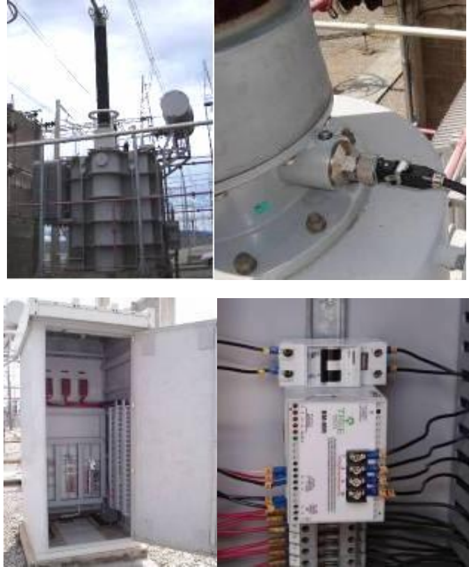
Fig. 4 – Details of bushing monitoring system installed [3]
