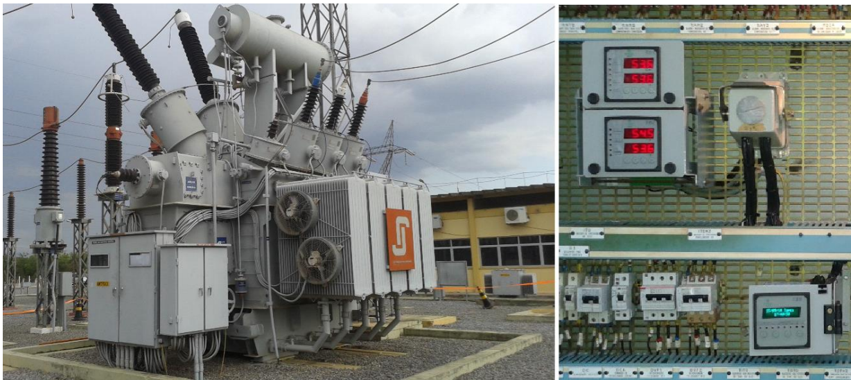
Figure 5 – Transformer at Nova Mutum SS and IEDs installed inside the panel
