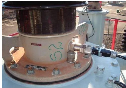
Figure 4– Direct connection of the monitoring system to the bushing tap of side [5]
