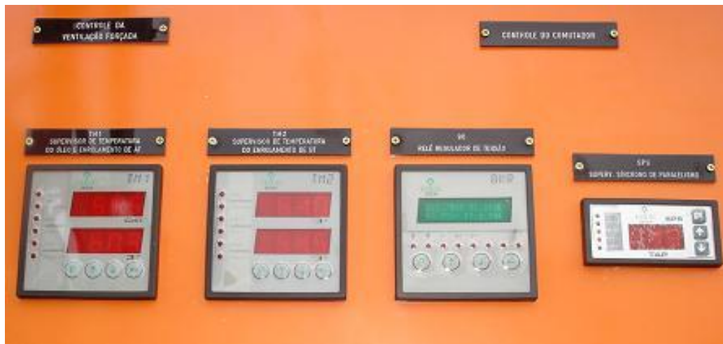
Figure 5 - Photograph of the Installed IEDs
