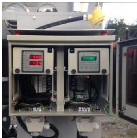
Fig. 05 - Temperature Monitors and Bushings
