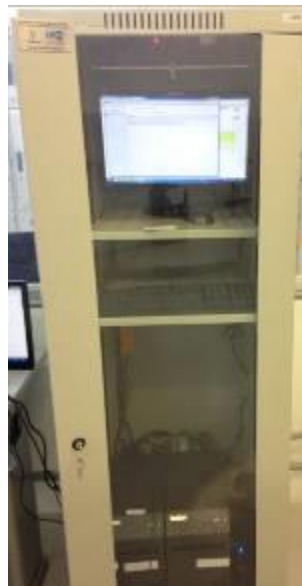
Fig. 03 - Data server with the online monitoring software;
